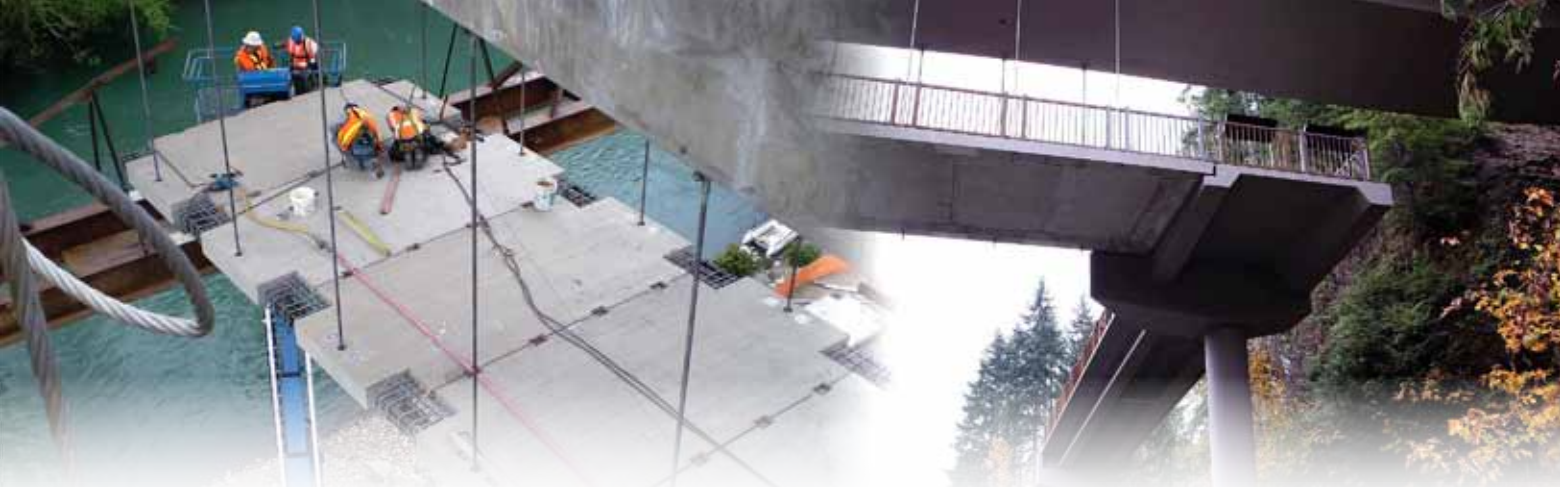
The pedestrian bridge features 56 precast concrete deck segments below the main bridge and four deck bulb-tee approach girders along the river bank to transition to the Olympic Discovery Trail.
